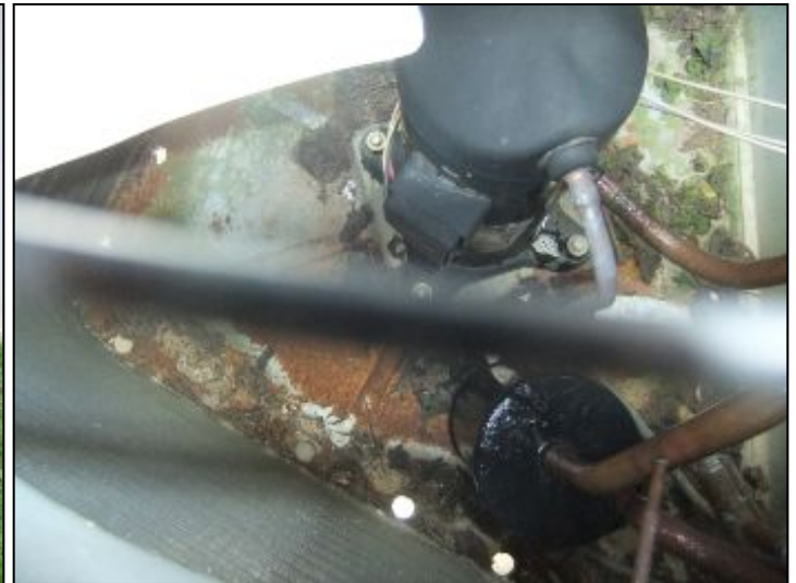
Inside a/c unit
