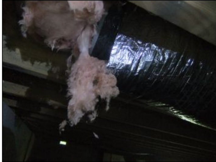
Boot insulation needs to be repaired
