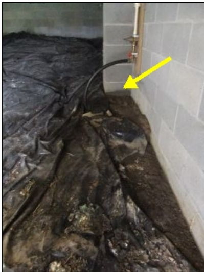
Lots of moisture on block and dirt
