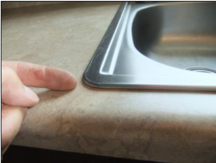
Sink is loose and has no sealant under rim
