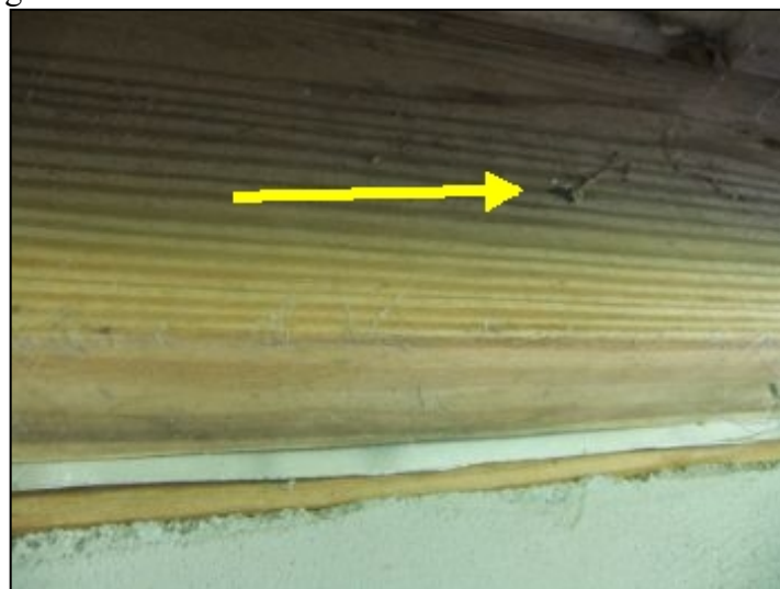
Ledger to house nails used instead of lag bolts. Add lag bolts or thru bolts.
