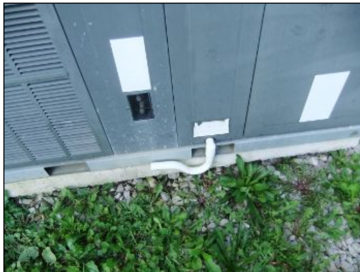
condensate line intact
