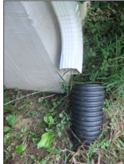
missing connector to drainage pipe
