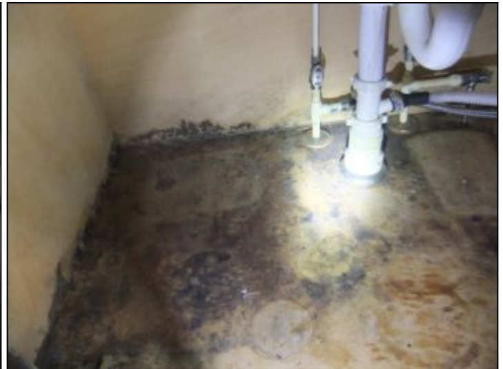
Mold in cabinet
