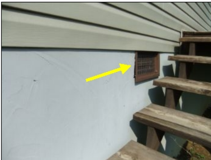
Vents are loose and can allow insects to enter crawlspace. Tighten and seal vents.
