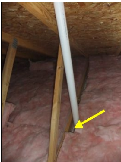
Missing insulation above master bath
