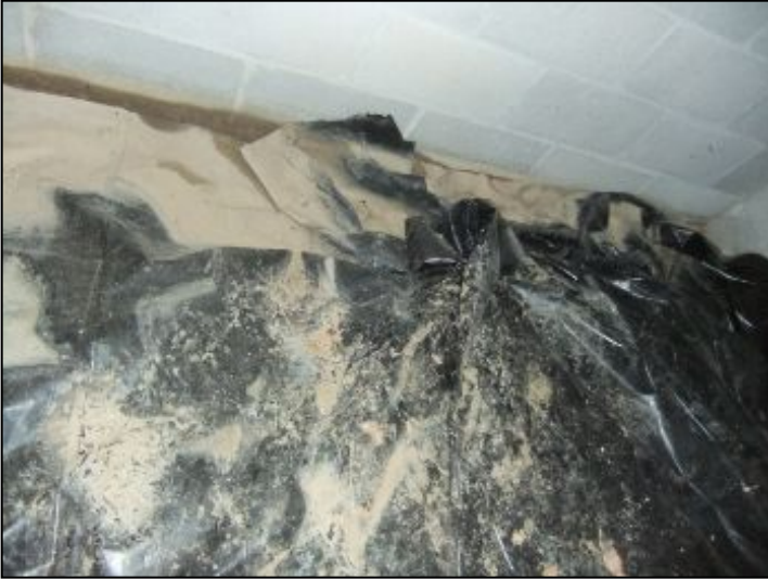
Signs of standing water at back of crawlspace
