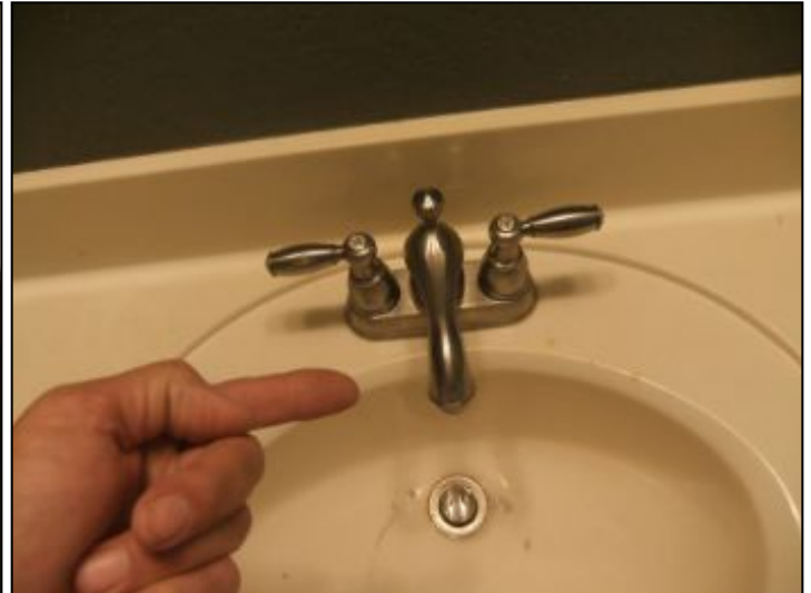
faucet needs repair
