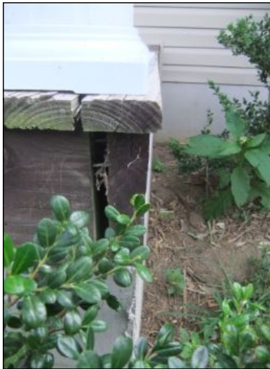
Rim board needs to reattached
