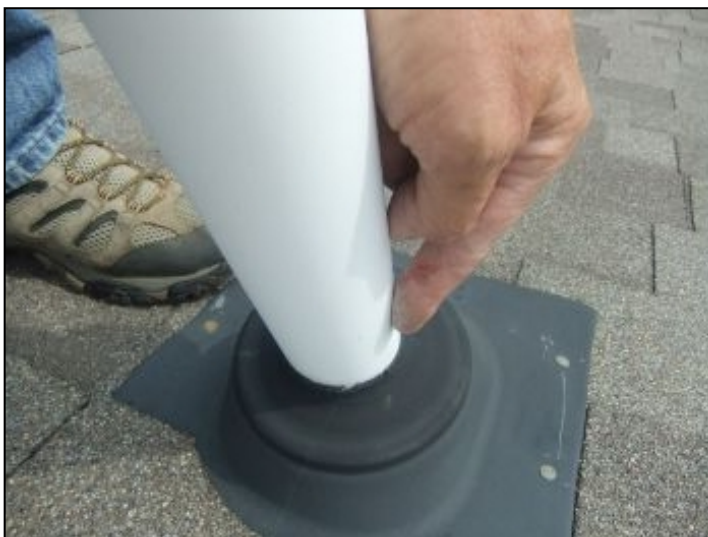
Missing clamp at boot #1
