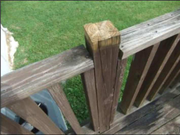
small nails at top of post need to be removed
