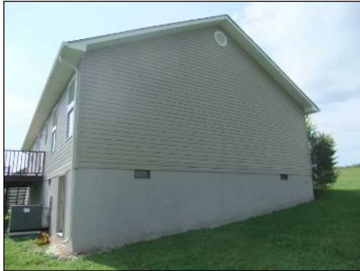
GROUNDS DRAINING AND GRADE CONDITIONS
