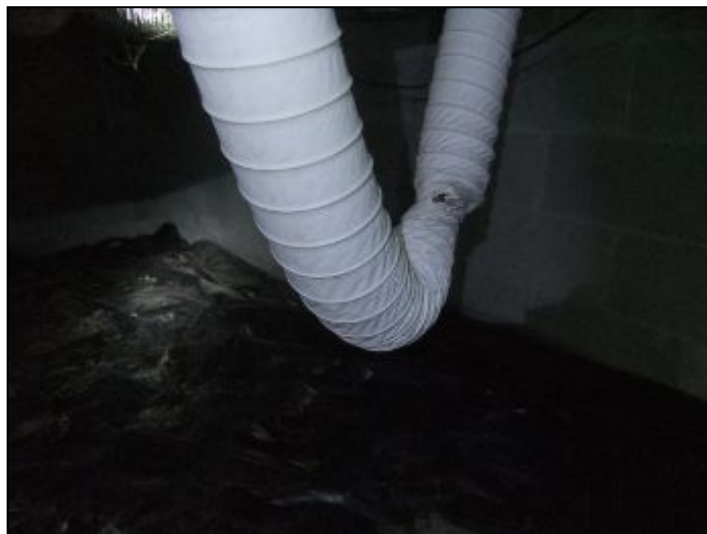
Dryer vent hose has hole. Replace with solid metal pipe
