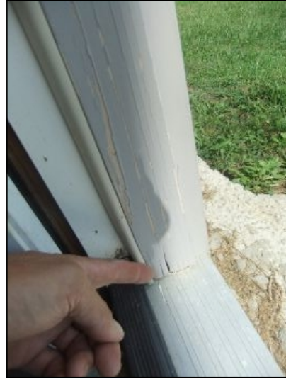
Jamb of access door needs repair
