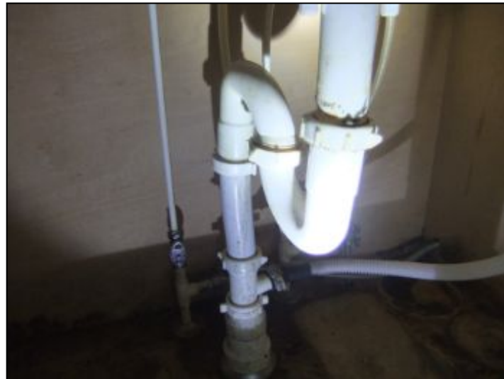
Drain used to be leaking here
