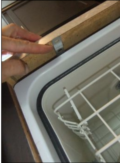
Dishwasher not fastened to countertop
