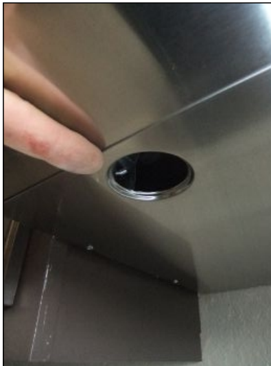
Missing light bulbs
