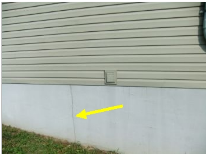
Crack in parge coating
