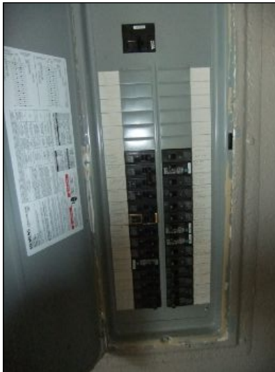
ELECTRICAL MAIN SERVICE CONDITIONS
