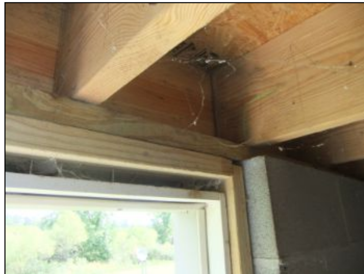
No beam above crawlspace access door
