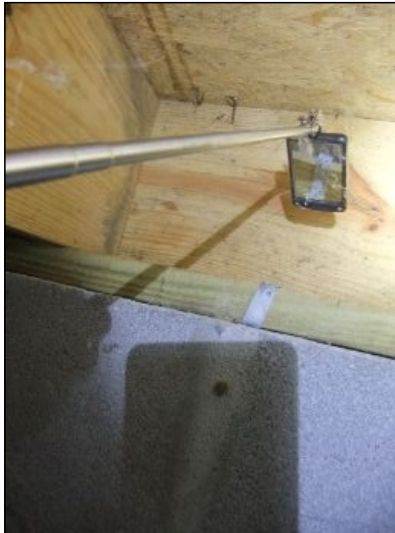
No nails in straps holding plate to block
