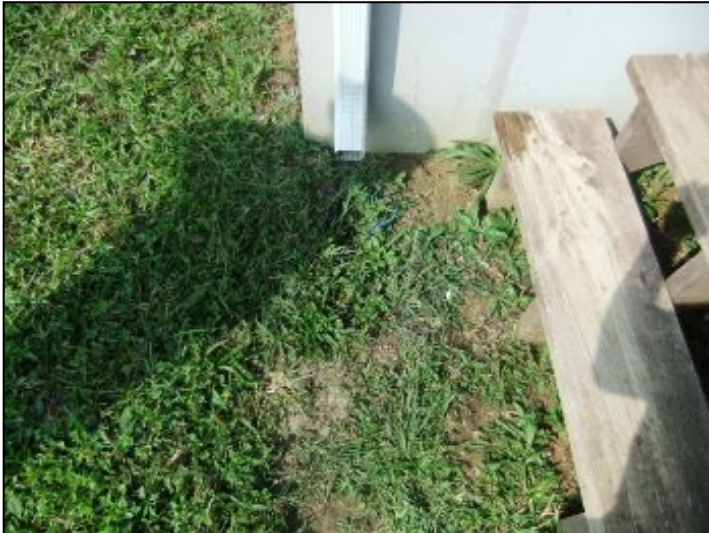
Downspout should be redirected away from bottom of stairs to eliminate slick or icy conditions.
