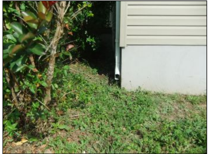
Downspout extension needed. Turn downspout so water flows away from house.
