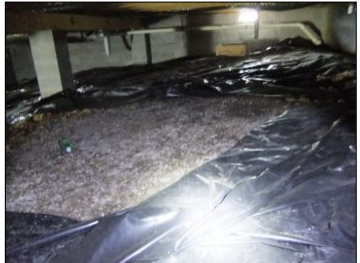
missing plastic sheeting
