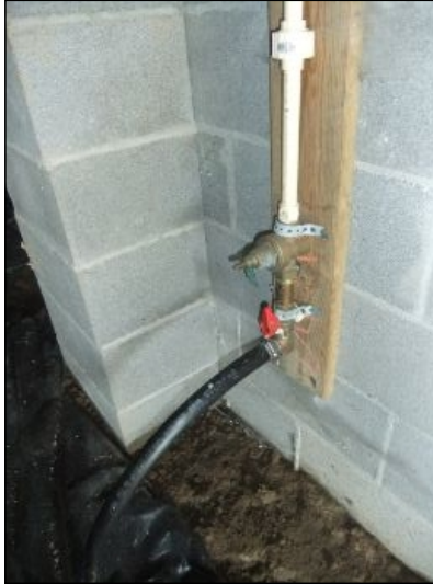
main supply with pressure regulator
