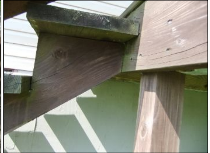
Stairs should have hanger attaching it to deck
