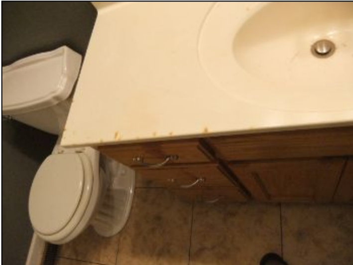
burn marks on sink top
