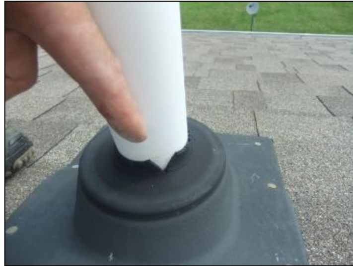
#2 boot starting to split and missing clamp
